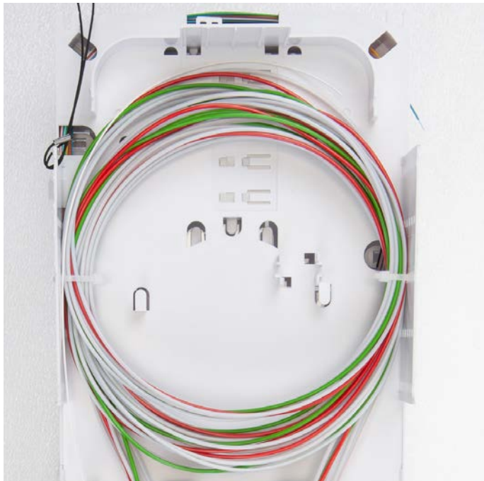
6.2.8 Loop storage, attach bundle to the sides with cable ties.
