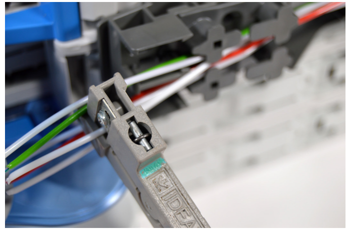
7.1.2. Strip the loose tubes at the marked point and clean the fibers.
